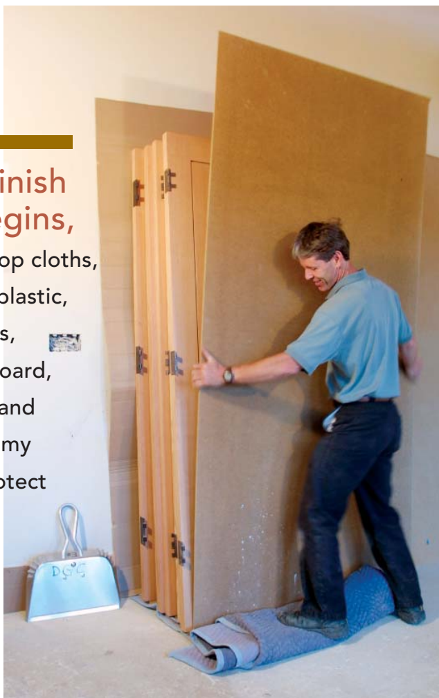
Putting the doors under wraps. After the doors are hung, they are removed, stacked away from high-traffic areas, and protected with moving blankets and fiberboard.
