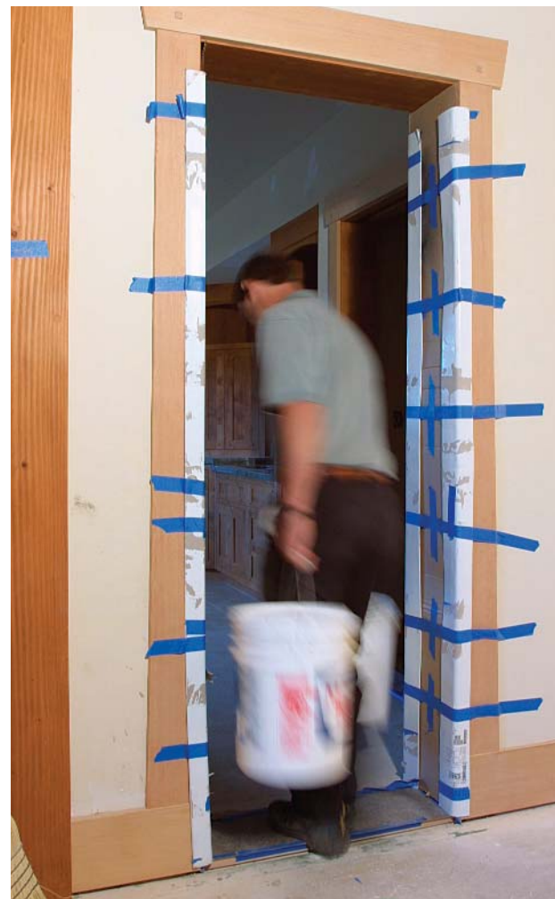
Protect doorways that are in the way. To keep door jambs free of nicks and dings, the author likes to wrap interior doorways with cardboard and blue tape. Exterior door jambs (and exposed beams) are armored with plywood.
