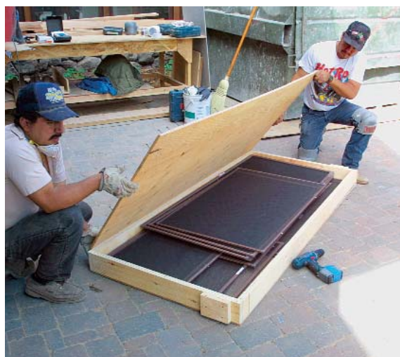
Site-built boxes protect screens. When the windows arrive on site, the screens are removed for safekeeping in plywood boxes built by the apprentices.
