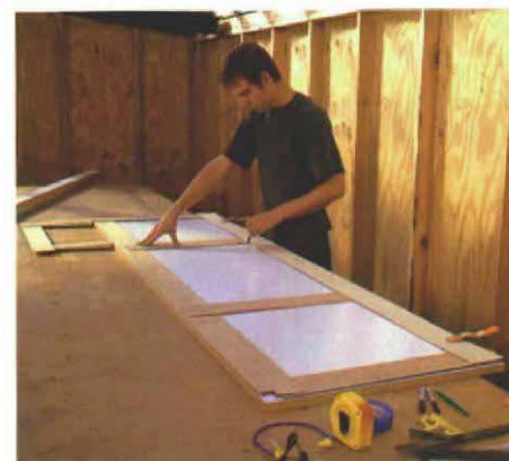
Template defines the countertop's shape. A template (top photo) made of thin plywood strips hot-glued together is an accurate means of transferring the shape of the counter onto the mold. After notations are written on the template indicating site particulars, the template is flipped over (remember, the mold is upside down), and the information is transferred onto the melamine blank (bottom photo).
