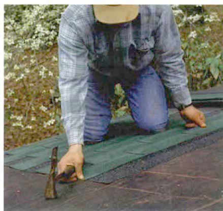
Running; straight courses. The author aligns shingles using a gauged roofing hammer and vertical bond lines.
